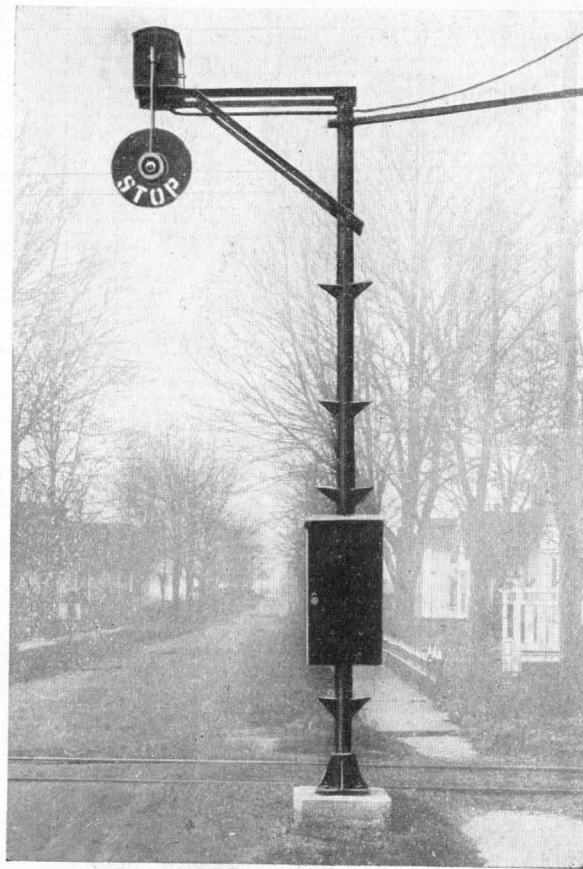
600-volt D.C. Electric Line Installation of Magnetic Flagman (two position, lower quadrant), on Interstate Public Service Co. at Scottsburg, Indiana.
