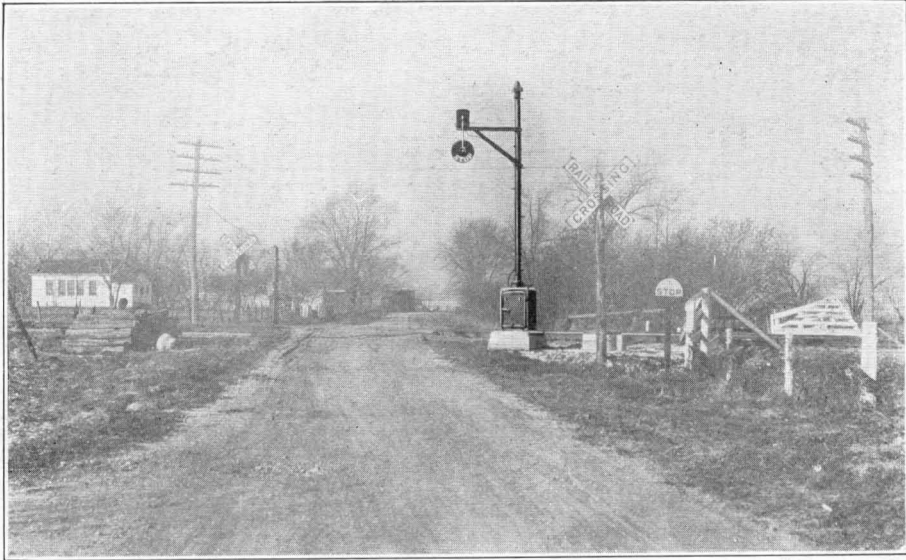
Installation of Magnetic Flagman (two position, lower quadrant), on the Atchison, Topeka and Santa Fe R.R. at Emporia, Kansas.
