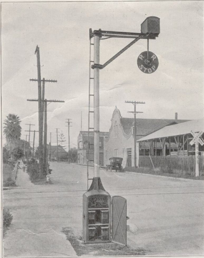
Magnetic Flagman installation on Southern Pacific at Anaheim, California. The above cut illustrates an 8-volt D. C. (Caustic Soda) Battery operation controlled by D. C. track circuits.
