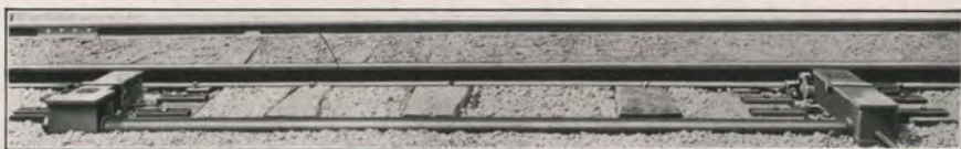
Track Instruments as Installed on Single Track to Give Indications for Trains Running from Right to Left
