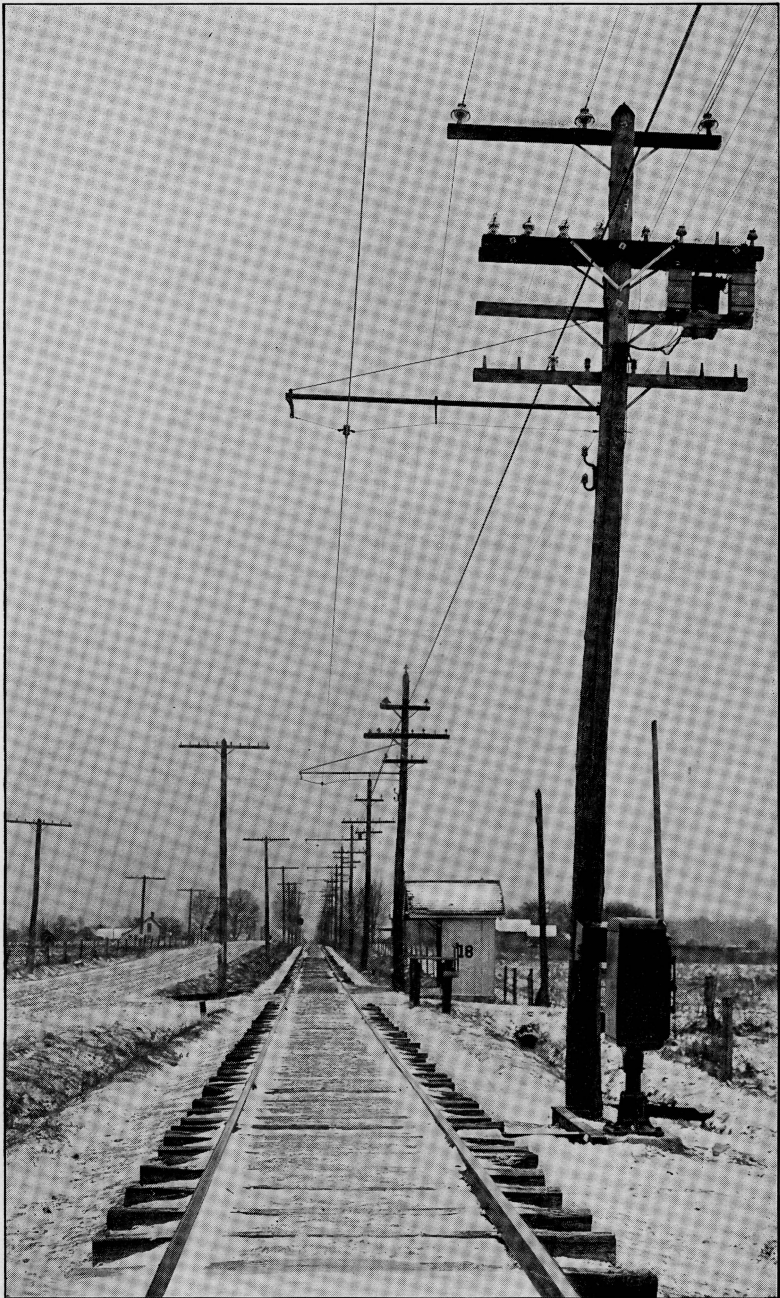
Transformer, High Tension Lightning Arresters, Lightning Arrester Box and Relay Box. Indianapolis, Columbus & Southern Traction Co. The TDB System.
