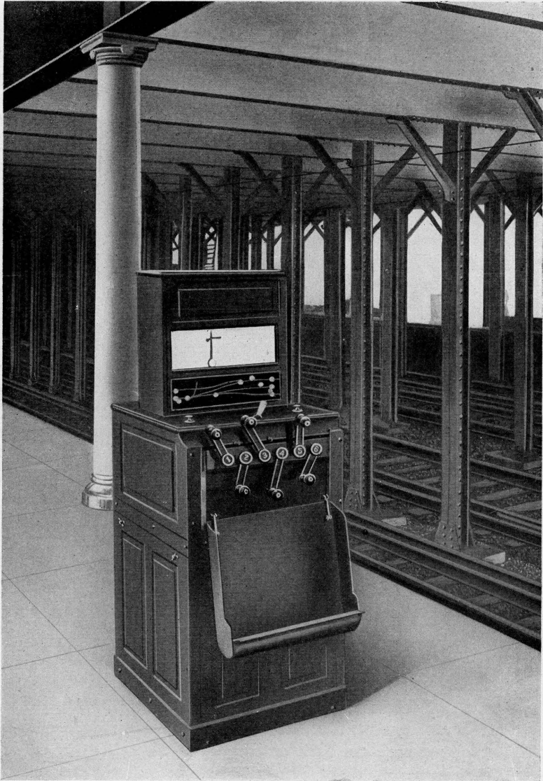
A TYPICAL ELECTRO-PNEUMATIC INTERLOCKING MACHINE LOCATED UPON A STATION PLATFORM, FOR THE OPERATION OF CROSS-OVER SWITCHES
