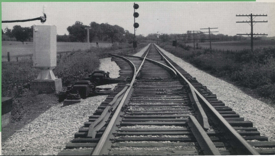
Switch Location, Remote Control Installation near Terre Haute, Ind. C. M. St. P. & P.—C. & E. I.
