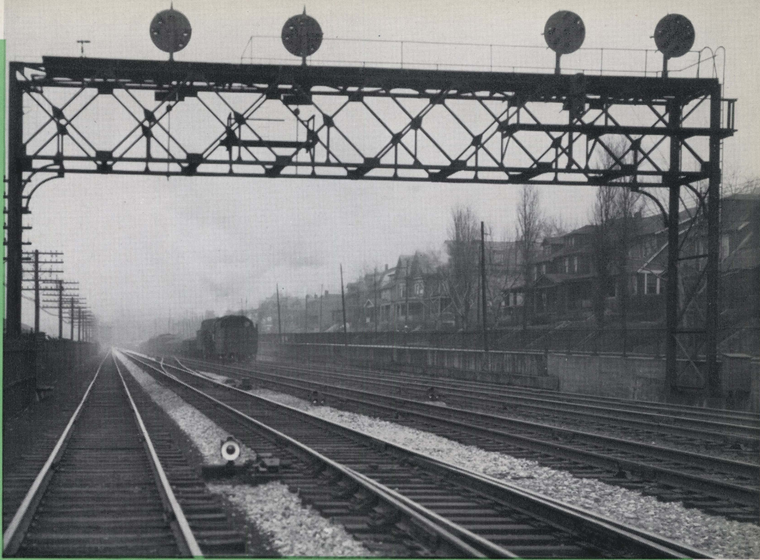
Remote Control Layout on Four Track Line Near Pittsburgh, Pa.—P. R. R.
