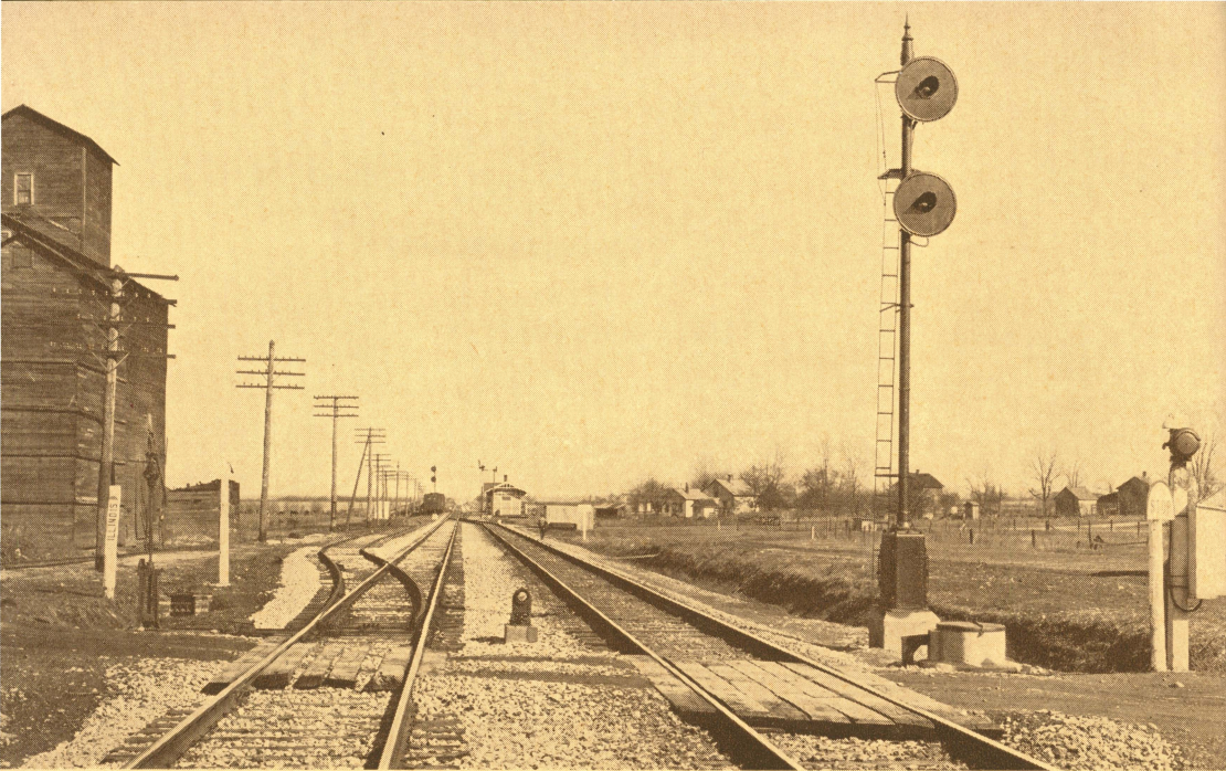
C. T. C. is Applicable to Long as well as Short Sections. This Location, at End of Double Track at State Line, Ind., is Controlled from Peru, 93 Miles away—Wabash
