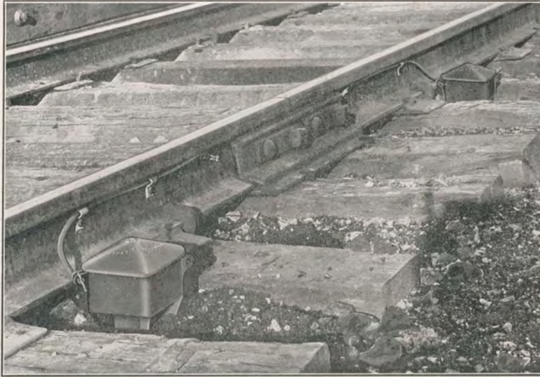
Bootleg Connections Using Model A-1 Parkway Outlets.
