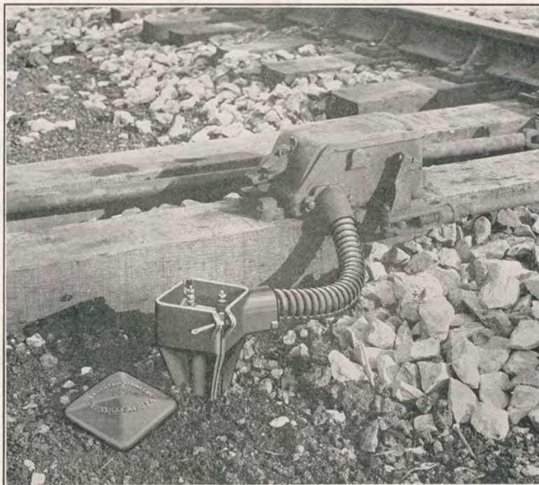
Model A-3 Parkway Outlet In Service at a Switch Circuit Controller.
