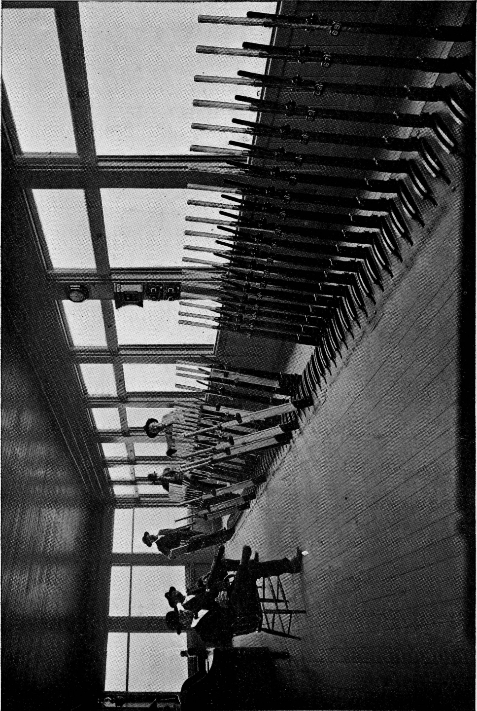
PLATE 9. Operator's Floor in Tower.
