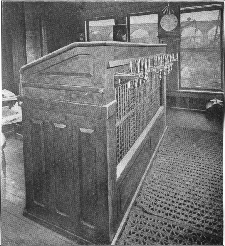
FIG. 21. ELECTRIC INTERLOCKING MACHINE.
