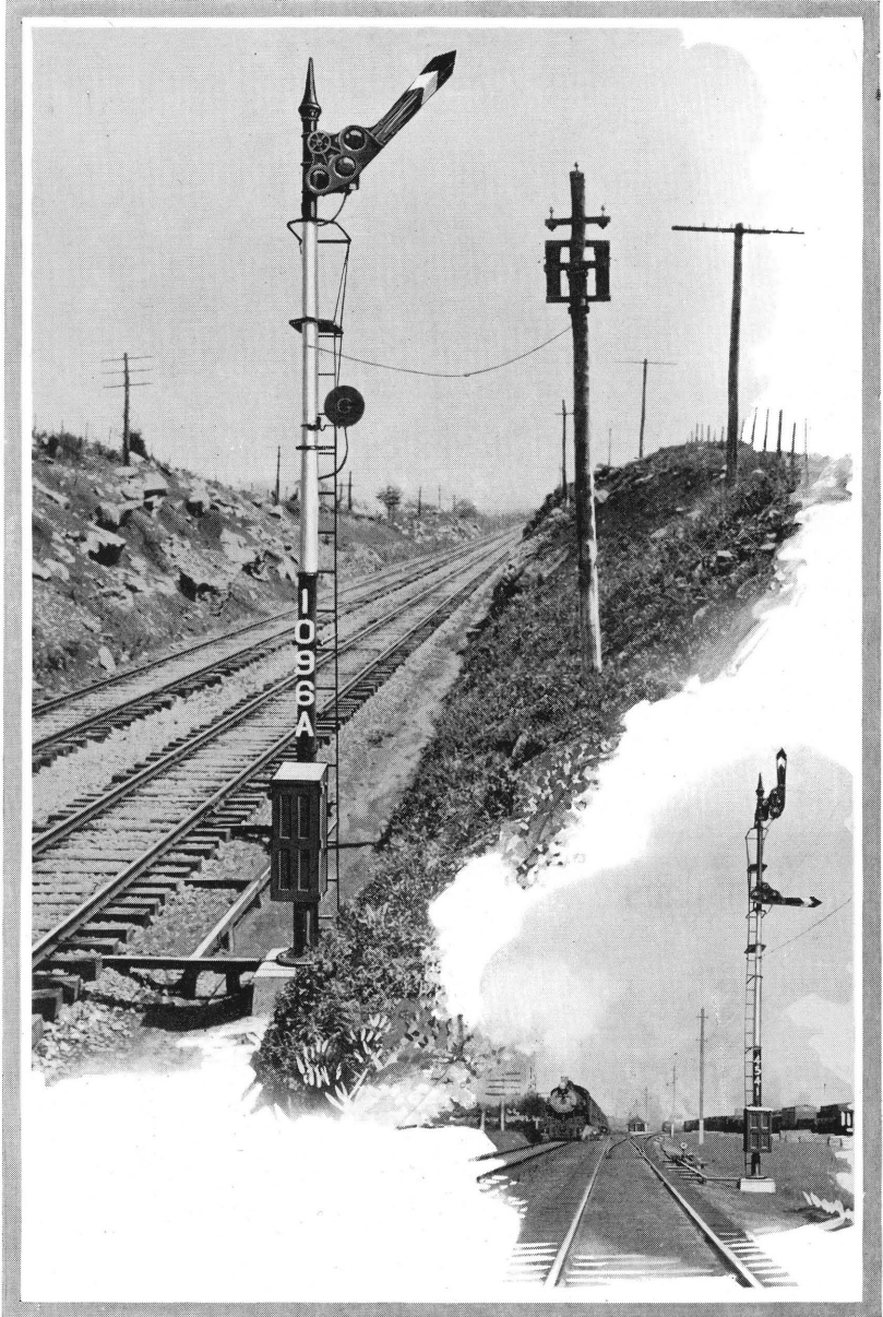
Fig. 2 a Grade Signal b Two Arm Signal approaching Station
