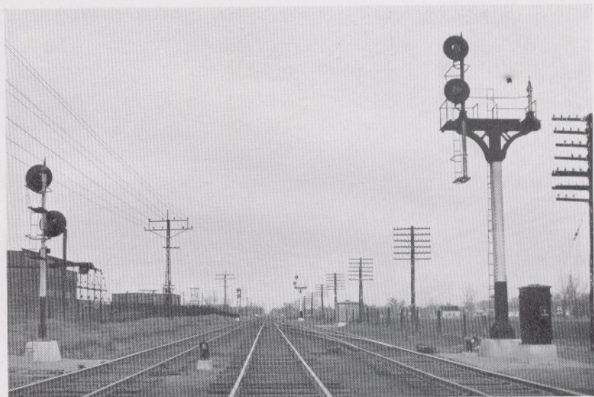
North Gate on the Albany to Watervliet, N. Y. (D. & H. R.R.) CTC Installation
